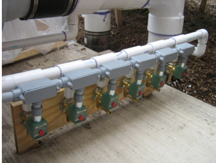
Figure 3-11 Solenoid Valve Sampling Manifold (Giant Eagle)
