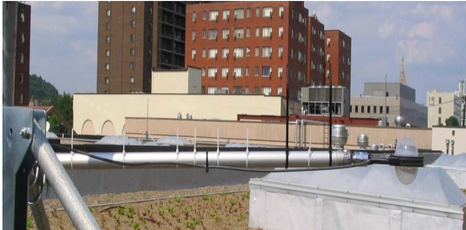
Figure 3-5 Net radiometer for measuring net radiation at the roof surface (Giant Eagle)
