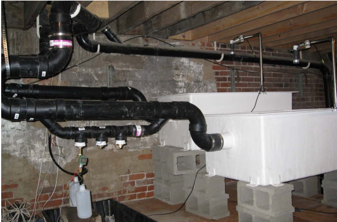
Figure 3-18 Drainage system at Homestead Site (located in the basement of the building). The weir next to the wall was used for the control roof and the other for the green roof.
