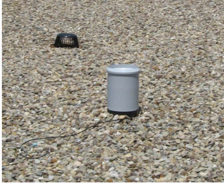
Figure 3-7 Rain Gauge Installed on the Green Roof (Giant Eagle)
