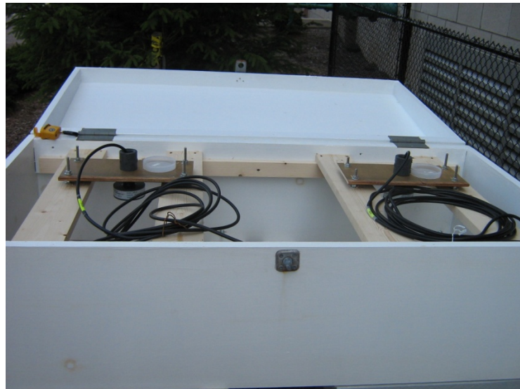
Figure 3-9 Ultrasonic sensors installed atop the flumes for measuring stormwater runoff (Giant Eagle)
