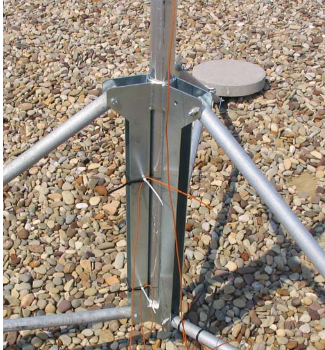
Figure 3-4 Thermocouple wire for temperature monitoring Attached to Tripod (Giant Eagle)
